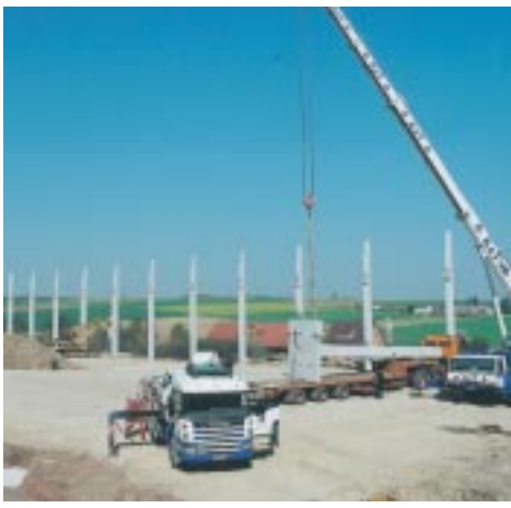
A milestone: construction of a new production hall with new foaming plant.
